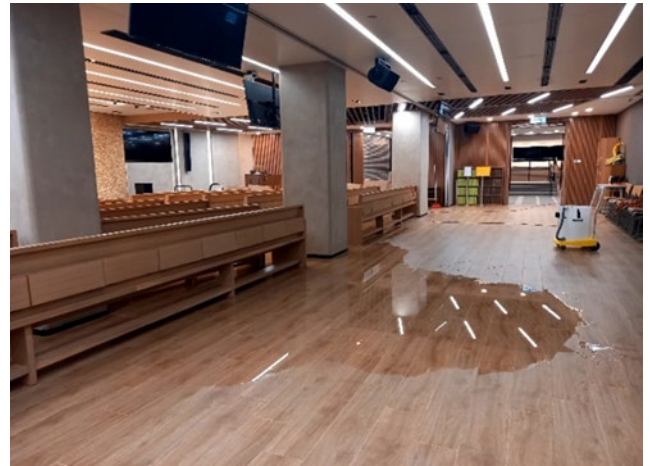
Water leakage from the stage podium to the back of the auditorium
